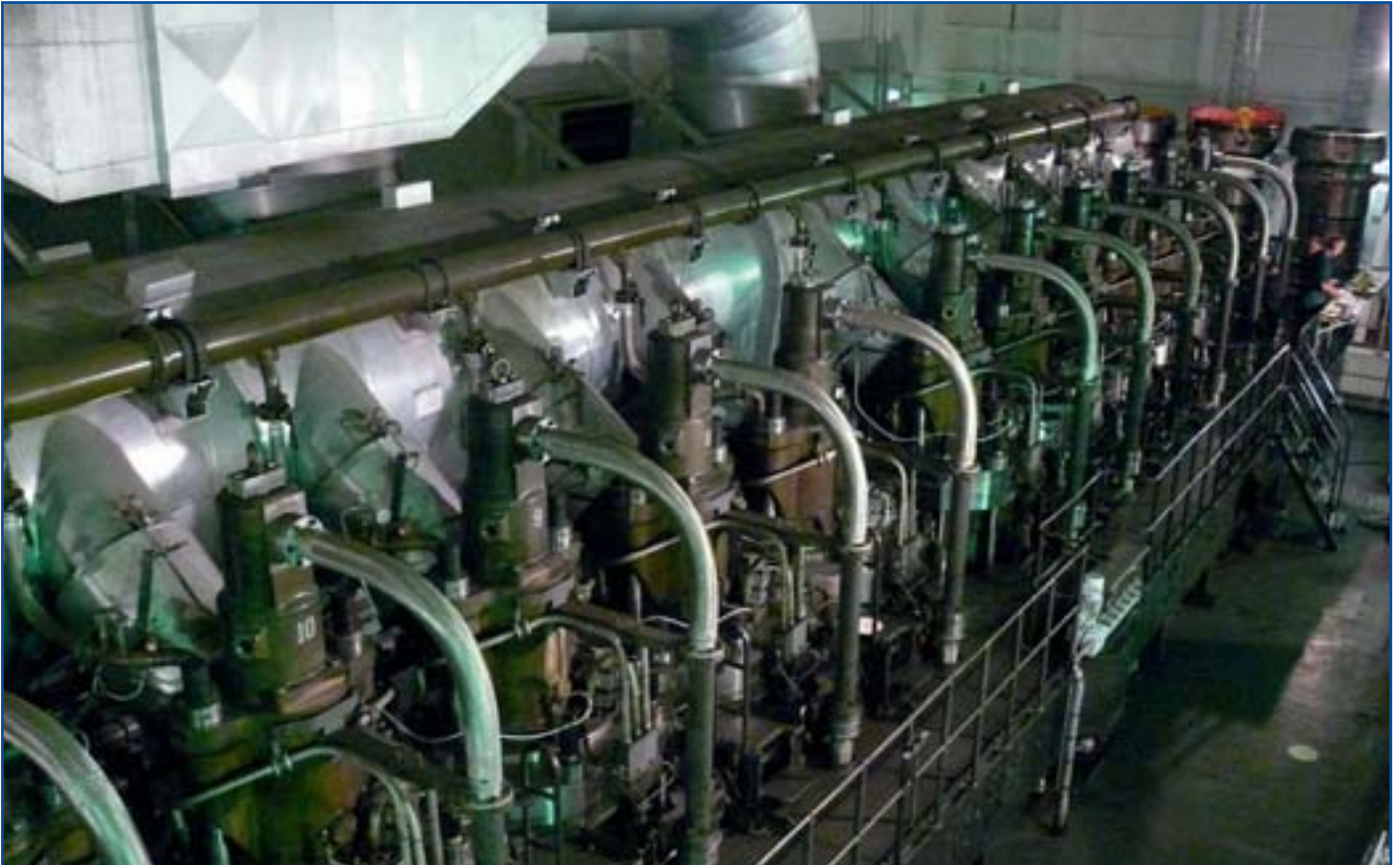
A number of accidents occurred during servicing and maintenance work
